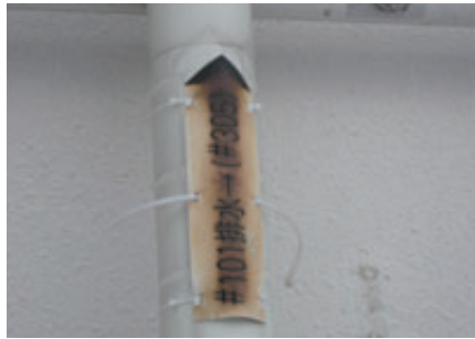
Example of recommendation Indication on piping has deteriorated, and needs replacing. (comment by an auditor)
