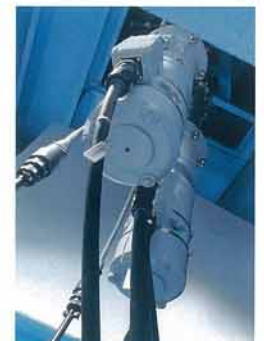
Installed S-FMCRD (test loop) ▲
